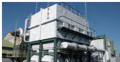
Dried-synthetic rubber waste incinerators at the Chiba Plant
