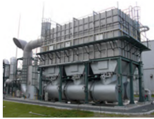
Dried-synthetic rubber waste incinerator (Kashima Plant)
