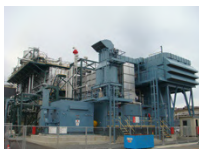
Natural gas-fired turbine cogeneration system (Yokkaichi Plant)
