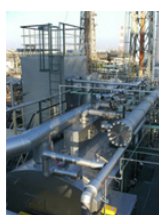
Sludge dryer system (Yokkaichi Plant)
