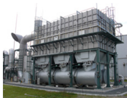
Dried-synthetic rubber waste incinerator (Kashima Plant)
