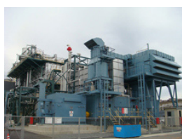
Natural gas-fired turbine cogeneration system (Yokkaichi Plant)
