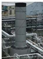
Ground flare (Yokkaichi Plant)
