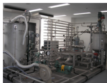
Miniature Plant in Yokkaichi Training Center
